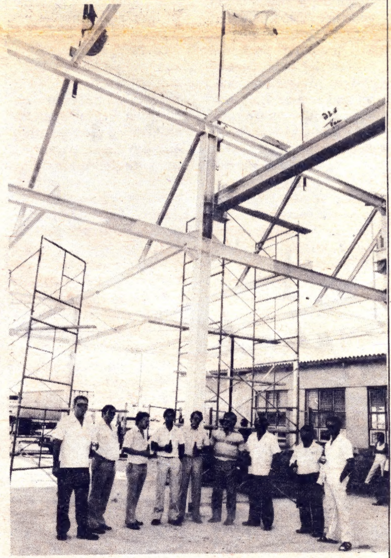
ORANJESTAD—Construction of the Aruba Ports Authority workshop reached its highest point on Friday, January 18. The building was started in September and is expected to be finished in May. Building contractor is ALBO n.v. and UNICON is in charge of the electrical installation. The workshop which costs about 900,000 guildres will house all the necessary machinery and equipment to service the ports of Aruba.
